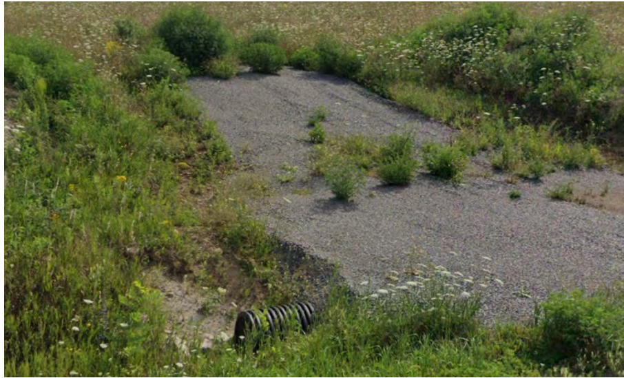
Image 11: One of two old driveways built over drainage ditch along Rosedale Road, view east.
